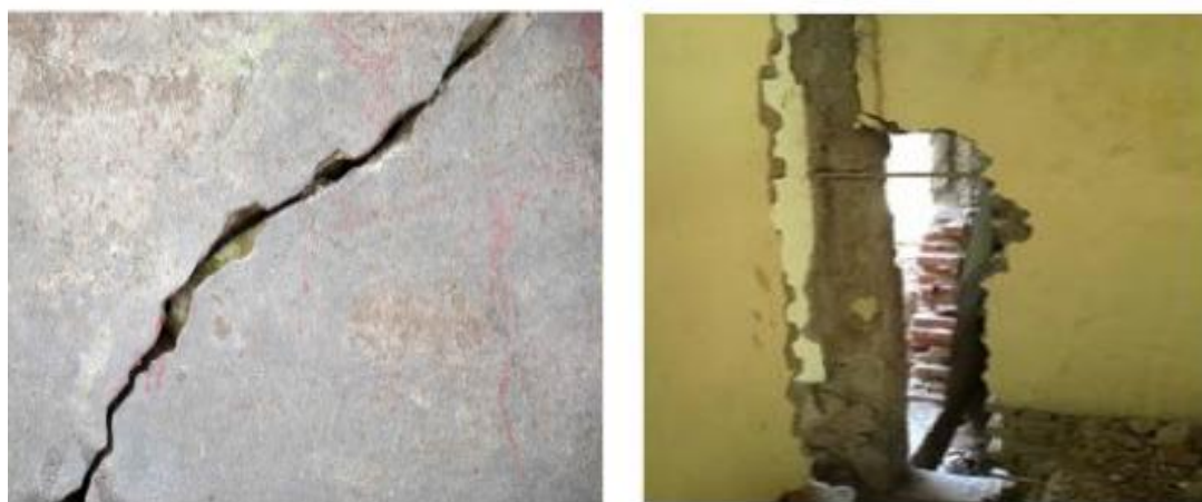
Fig. 1: Images of wall cracks in buildings
