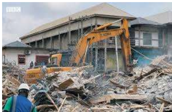
Fig. 7: Onitsha Shopping Plaza Collapse
