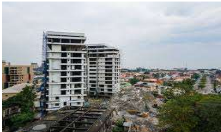
Fig. 5: Ikoyi High-Rise Collapse
