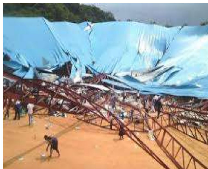
➤ Fig.6: Reigners Bible Church Building Collapse in Uyo, Akwa Ibom State
