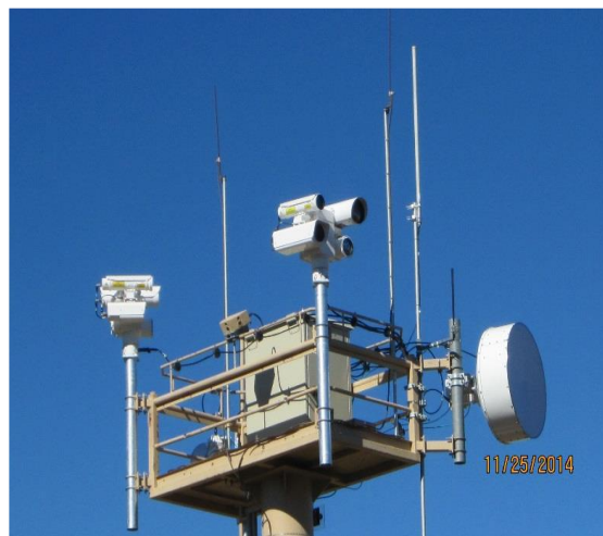
Fig 2: Remote Video Surveillance System (RVSS)
